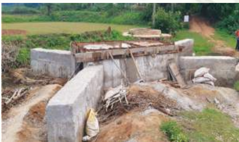
Culvert Construction at Tentuli VSS of Angul Division through convergence with RD Dept.
