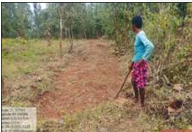
Fire Line creation work at Panasuan ANR plantation site in BJP FMU of Keonjhar Division
