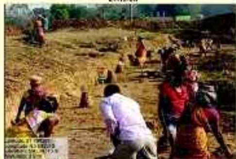
Pond Renovation work in convergence with PR Department through MGNREGS, Sankhapal VSS, Keonjhar Division
