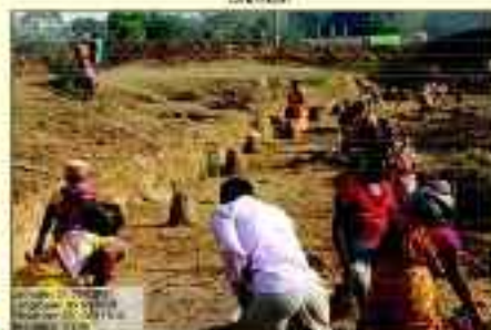
Pond Rehabilitation work in convergence with PW Department through MGNREGS, Sandilapat VSS, Nayagarh Division
